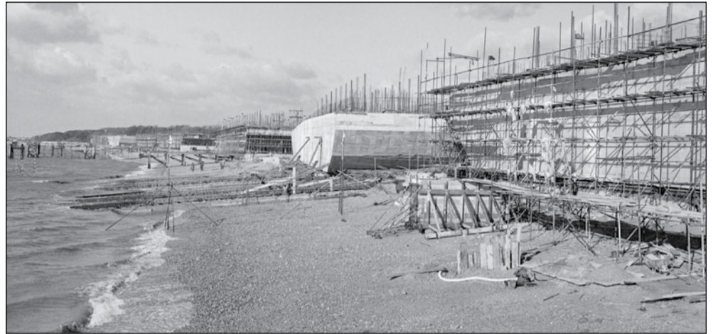
● Phoenix units under construction at Stokes Bay in Gosport, on the Solent, using hards which would later be used to load troops and vehicles on to landing craft
