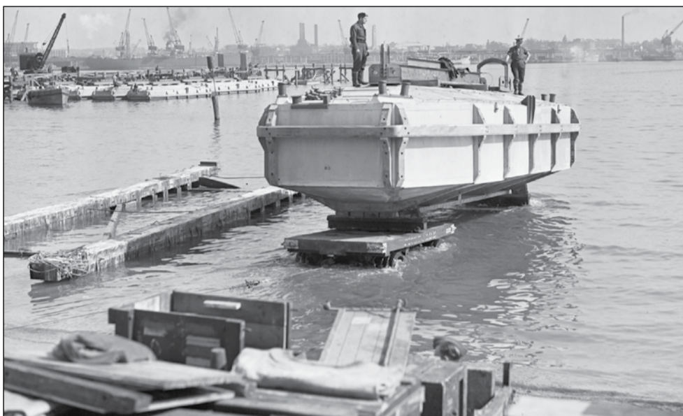
● A Beetle concrete float is launched, probably at Weymouth in Dorset or Marchwood on Southampton Water
