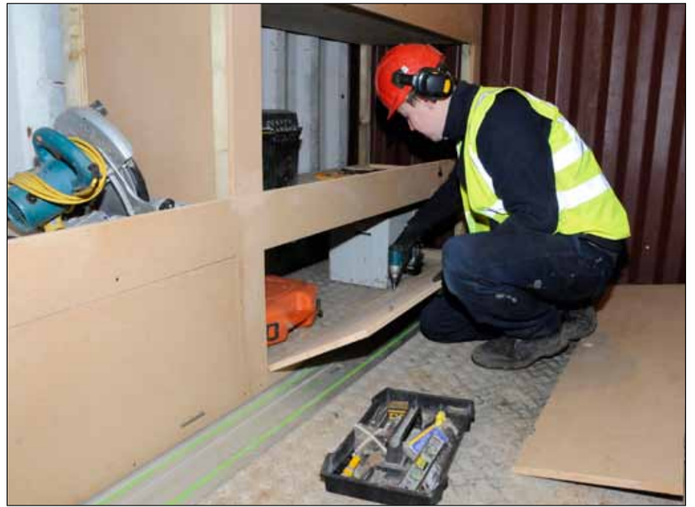
● A carpenter fits out one of the facility's mock bunk spaces featuring numerous hiding places
