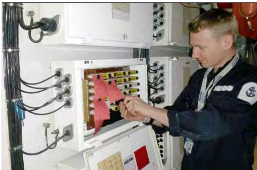
● LET (ME) Alan Wormald works on a fuse box onboard HMS Sutherland
