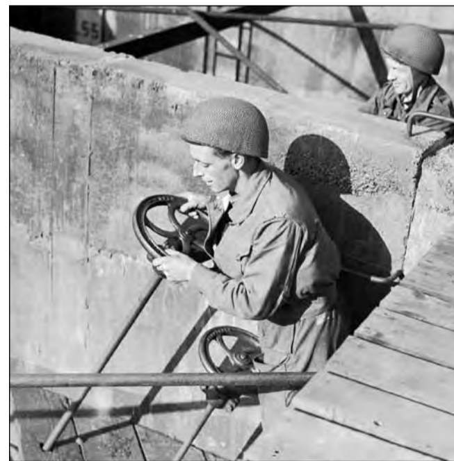
● (Above) Royal Engineers – Sappers – operating the valves of a Phoenix caisson to submerge it after it has been placed in position
