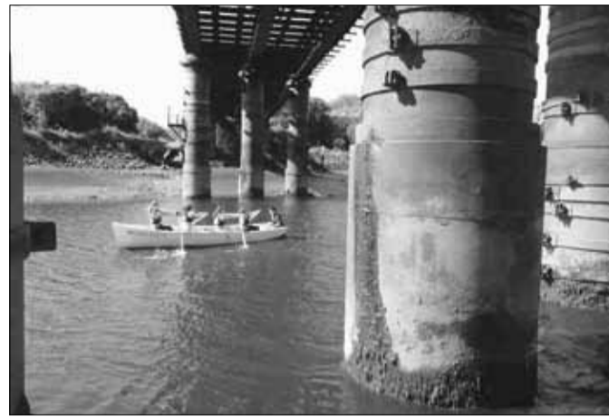
● Northumberland Sea Cadets pulling in a Trinity 500 boat on the River Tyne below the disused Scotswood Railway Bridge
