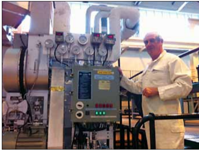
● One of two new vapour generators installed at HMS Sultan
