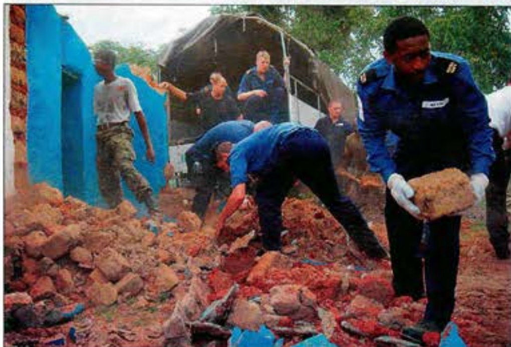
● NA Neil Wilson of HMS Albion clears rubble from a wall in Tokeh village
