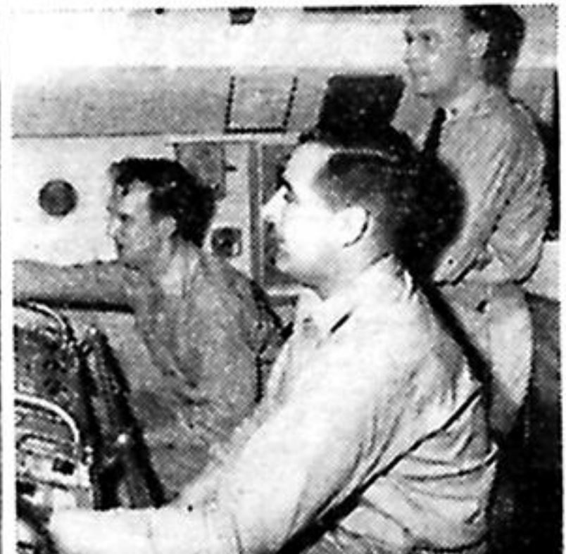
In the manoeuvring room of Skipjack, E.R.A. Flavell at the Reactor Control Panel, E.A. Shaw at the Electrical Control Panel with Cdr. Samborne as Engineer Officer of the Watch
