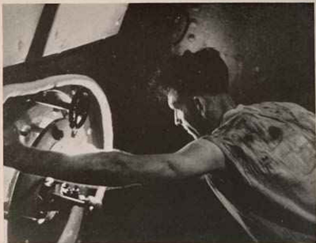
Lighting up a boiler
