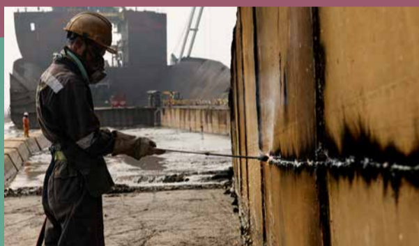
WELD WELD WELD: A Welder dismantling part of a ship during HMS Tamar's trip to the Peace, Happiness and Prosperity Shipbreaking Yard
